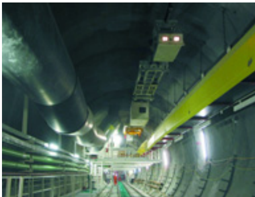
Monorail suspended from the tunnel roof
