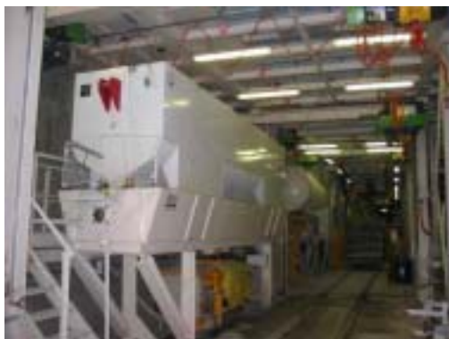
Transloading and intermediate stockage of pearl gravel (17 m 3 ) for the back-filling of lining segments
