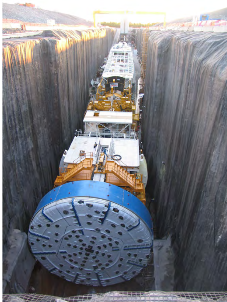
Picture: Overall view of back-up system
