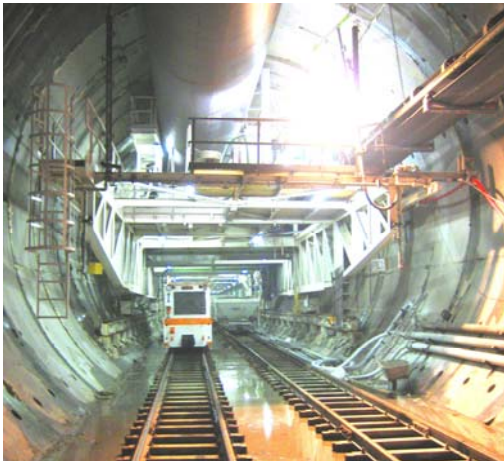
The back-up system is fit for double-track passage over the entire length of the train station. Thereby both, the heading supply as well as the invert lining supply, are equally ensured.
