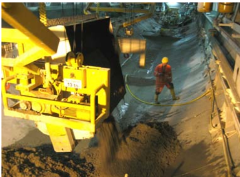
A high performance transloading crane with basket discharge installation (360°) supplies the floor lining construction site with fresh concrete.
