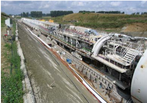
Back-up installation in front of the Section
